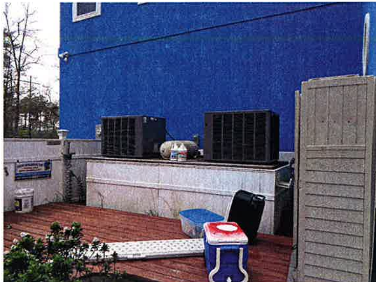
A/C UNITS - PICTURE TAKEN 03/17/2016
