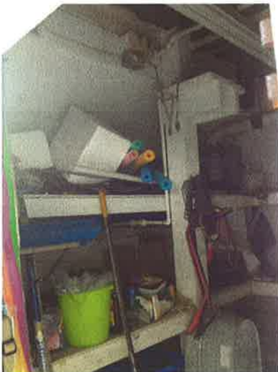
Electrical outlet in enclosure lower level. 03/27/15
