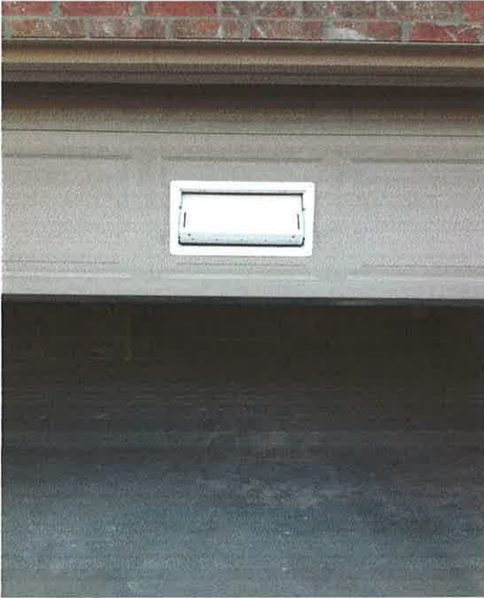
Garage door flood vent, Lot 25 Cypress Creek Ph 4, 12/13/12
