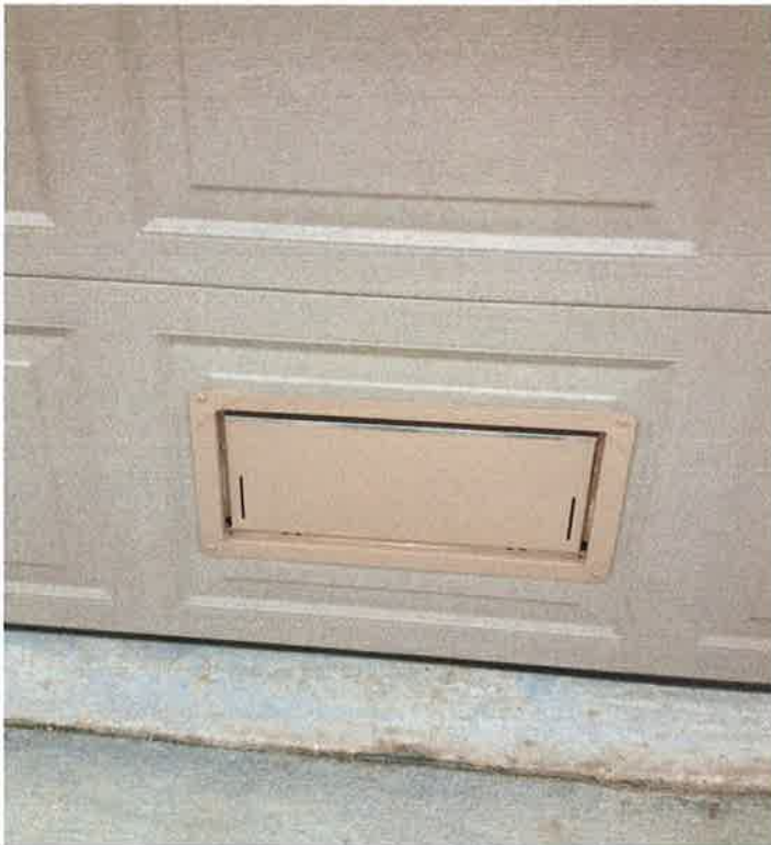
Garage door Flood Vent Lot 26 Cypress Creek, Ph 4: 2/4/13
