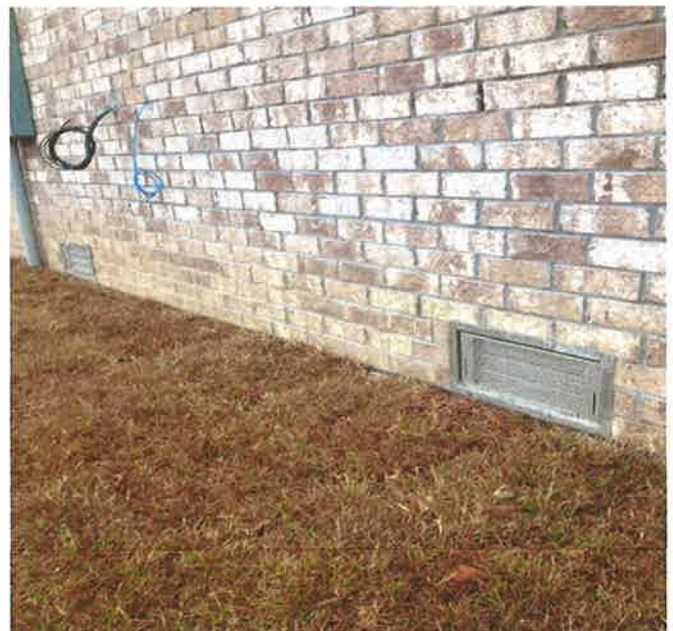
Garage wall flood vents Lot 26 Cypress Creek, Ph 4: 2/4/13
