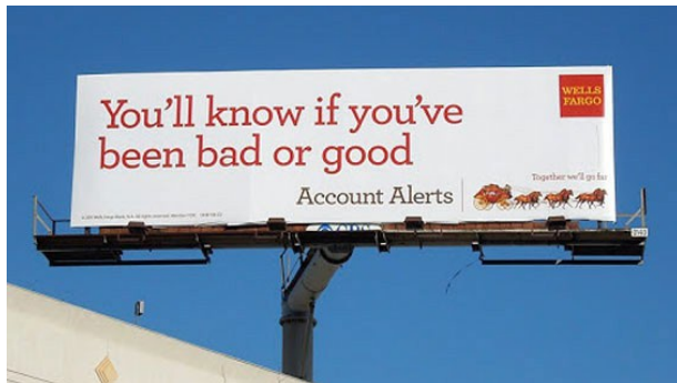
Billboard with a telescoping horizontal member resulting in sign being off center of the vertical support structure.
